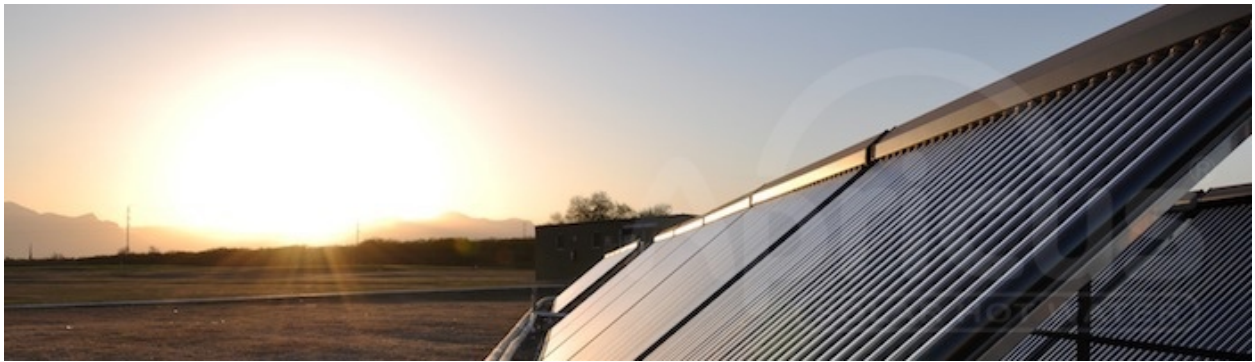
SOLAR THERMAL PANELS ON ROOFTOP
